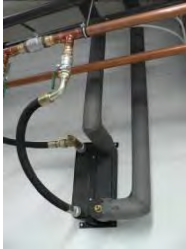
heat recovery from printing machine
