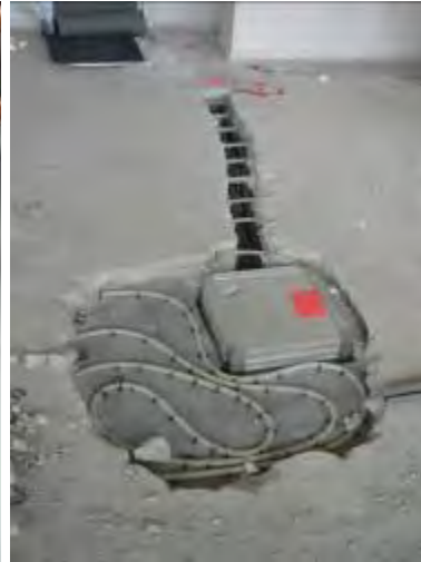
floor heating system
