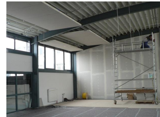
Upper floor with suspended cooling panels w/ integrated PCM.
